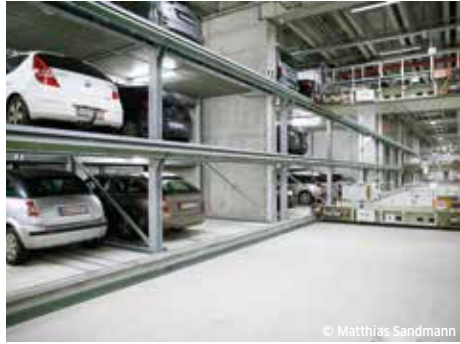
DOKK1, AARHUS Fully automated car park system with nearly 1,000 parking places
