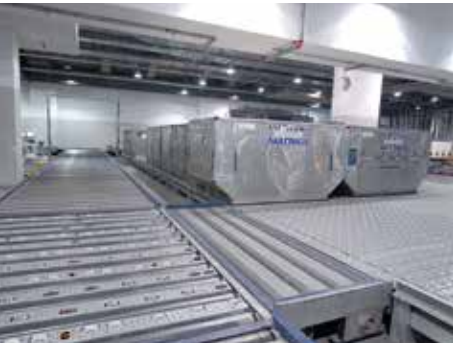
ASIA AIRFREIGHT TERMINAL T1 & T2, HONG KONG Air cargo system
